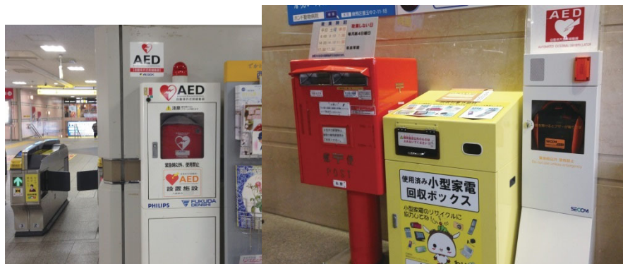
Fig. 13.7 Examples of Installed AED Boxes (Ministry of Health, Labor and Welfare, 2015)
